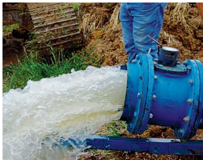
Figure 3. A 20 ML/day pump was used to generate 'fast' flows so that fast watering could be investigated at Bryandra, Katamatite.
