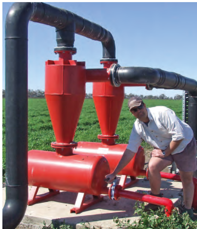
Heath Estens at the bore and filtration site, which will supply water to a high-tech irrigation system that has been installed to maximise water use efficiency.
